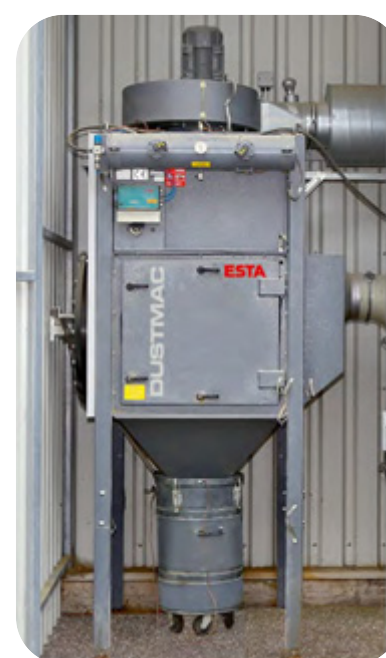
Central welding fume extraction system DUSTMAC F in the chemical industry
